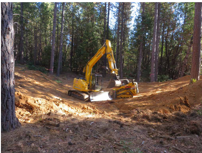
Heavy equipment used – an excavator and a Skidsteer digging an ephemeral wetland.
