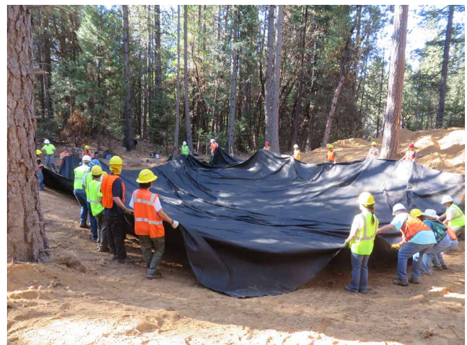
Class is laying-in what will be 3 layers of geotextile liners for the ephemeral wetland.
